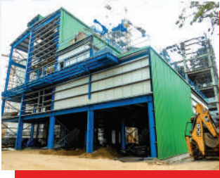
Power Plant Sri Lanka
