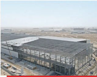
Cold Storage United Arab Emirates
