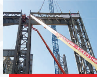
EOT Crane Unit United Arab Emirates
